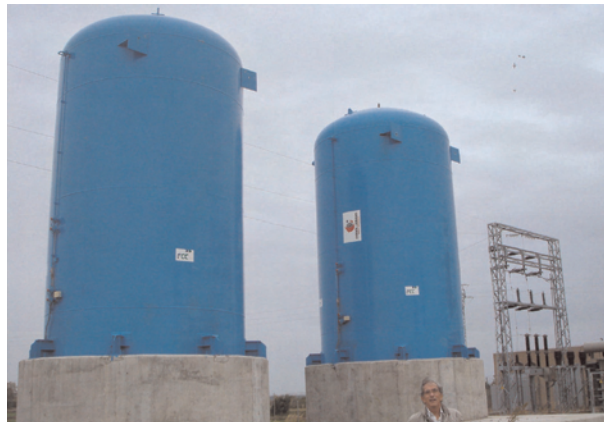
Fig. 5. Calderines de la central/ Surge tanks at the pumping station.
