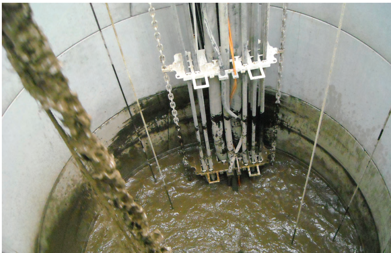
Fig. 7. "VSM" inundada trabajando/ "VSM" flooded whilst working.
